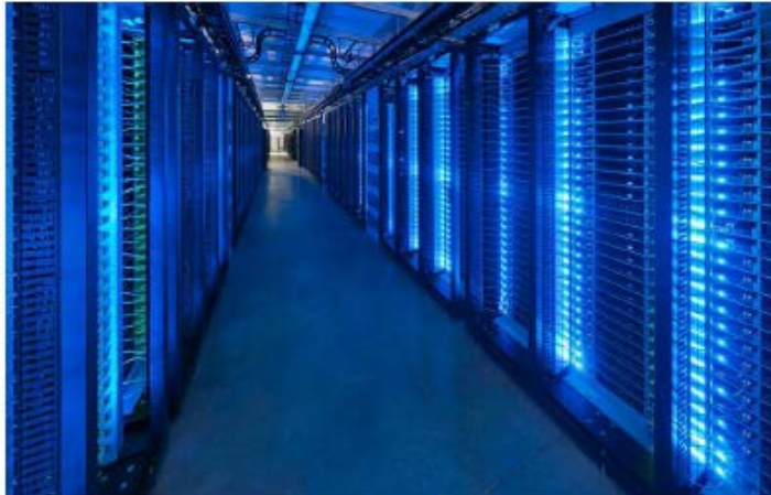
Data centers require non-stop electrical power
