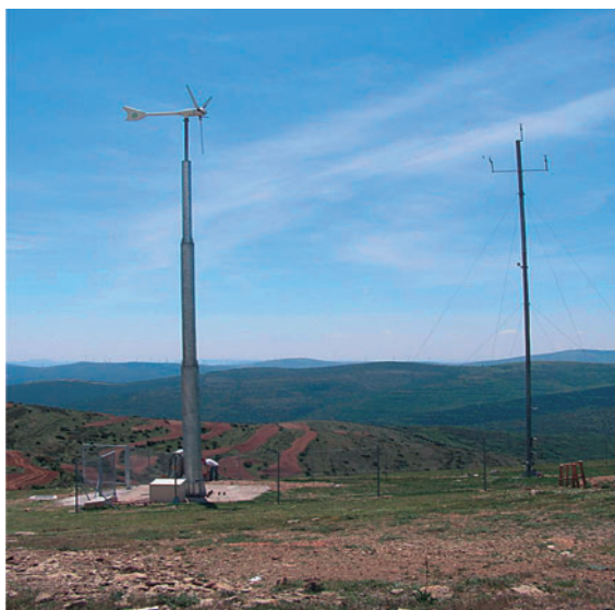
Figura 5. Aerogenerador Windspot 3.5 kW (SONKYO Energy). Fuente: CIEMAT.
